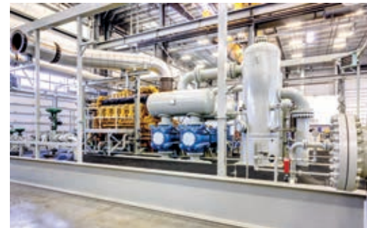
Compass is known for its compressor packages, such as this 3750 hp (2796 kW) package.
